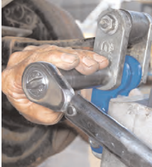
It's absolutely necessary to make sure all bolts are torqued to the manufacturer-recommended settings.
