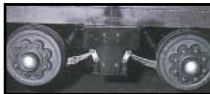
The stock shackle mount (top) is removed and the RE System (bottom) is welded in place. The system consists of a rubber block fused to a pair of steel plates; one plate mounts to the frame, the other is part of the moving suspension component.
